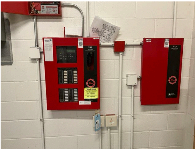
21 - FIRE ALARM PANEL
